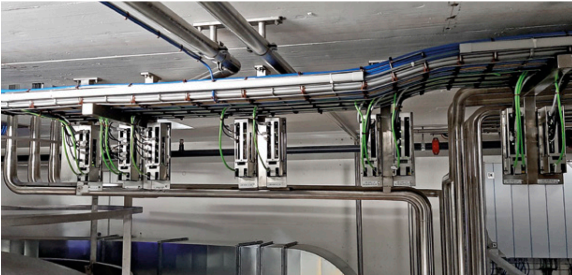
The TBEN I/O block modules are installed under the cable trays in ATEX protective housings to save space
